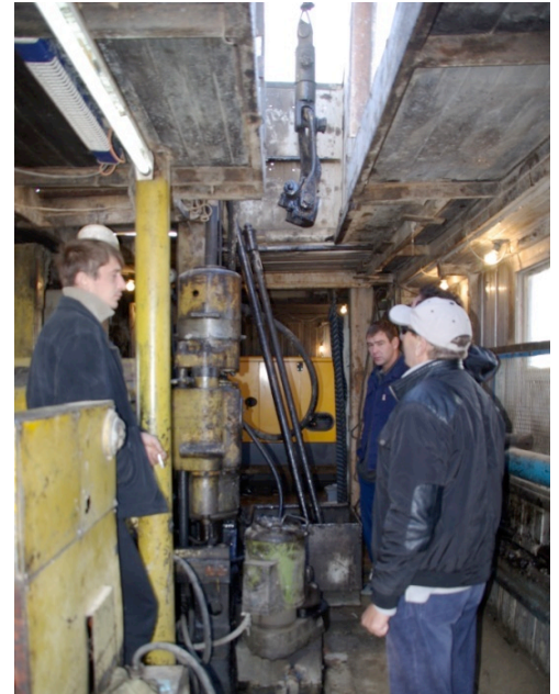
Drill Rigs used by CVR are built within caravans and are capable of working throughout the winter
